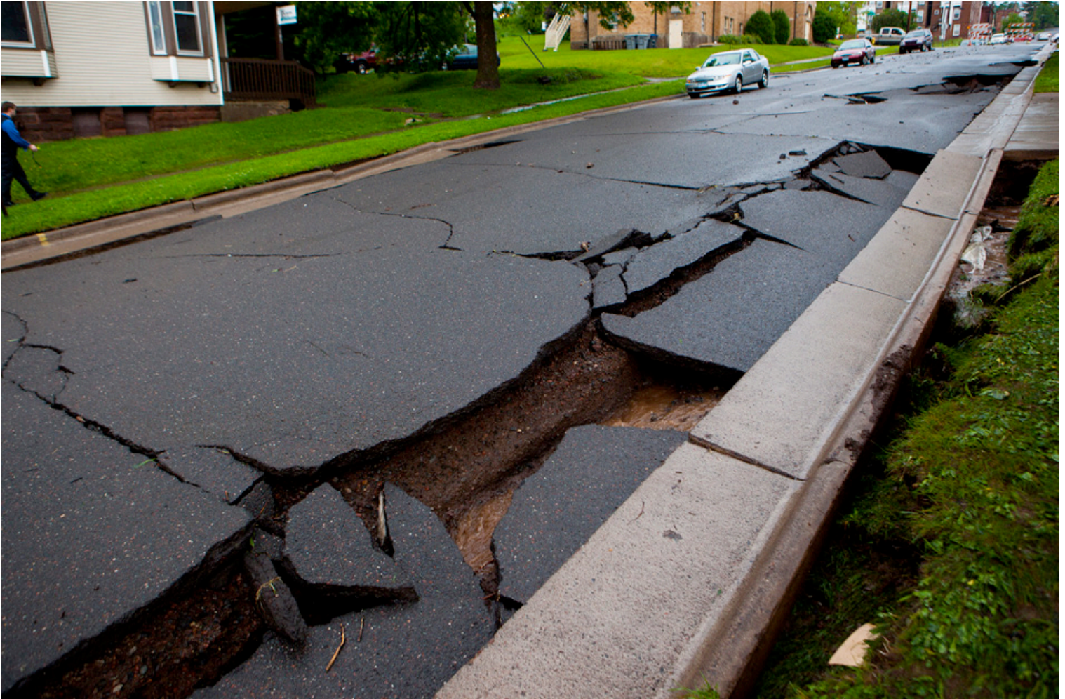
Duluth, Minn. — Portions of Seventh Avenue East in Duluth, Minn. collapsed Wednesday morning after heavy rains caused flooding. (Derek Montgomery for MPR) ( Read more about the flood ) LINK TO THIS PHOTO
