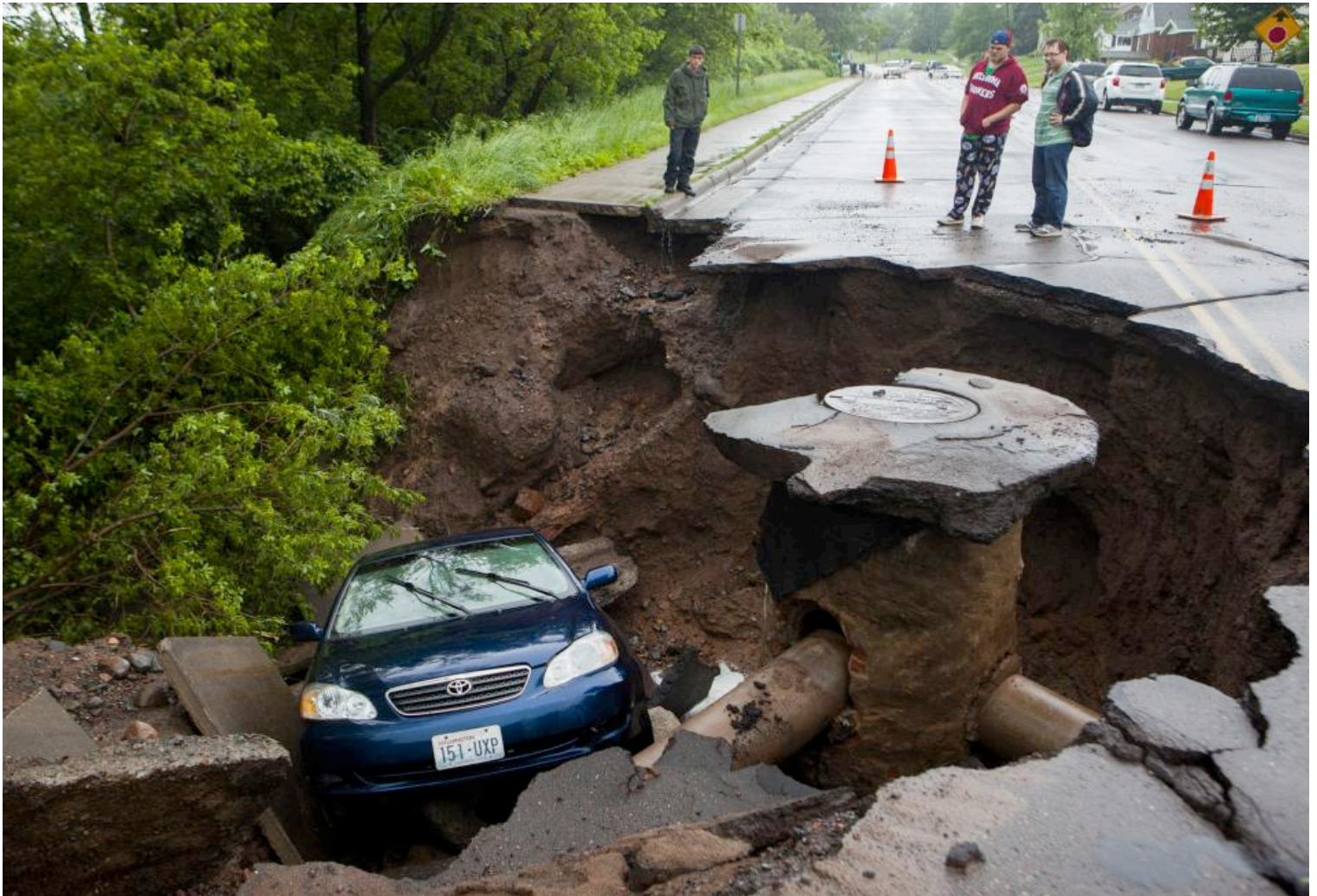
Duluth, Minn. — A giant sinkhole along Skyline Parkway near Ninth Avenue East captured this car Wednesday morning after heavy rains caused flooding in Duluth, Minn. (Derek Montgomery for MPR) ( Read more about the flood ) LINK TO THIS PHOTO
